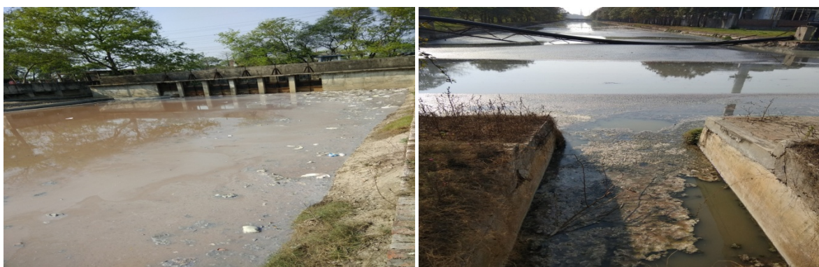
Fig. : Drainage outlet (Full of pollutants)
